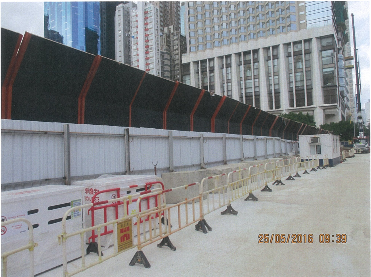
Photo 4A-2 Temporary noise barriers (western portion) for the construction of ADB (by Contract No. HY/2009/19)
