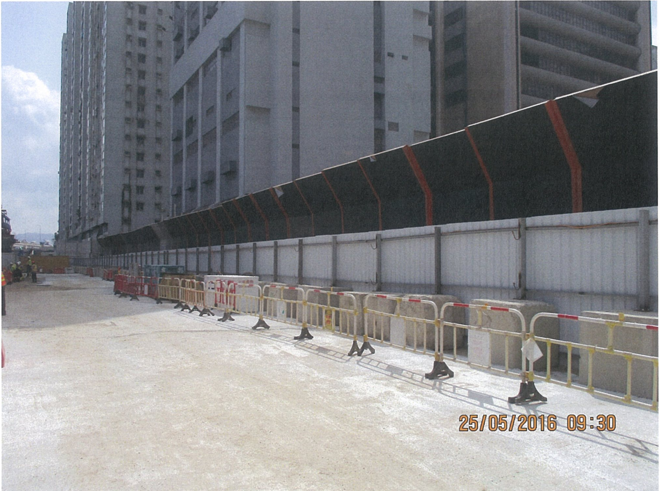
Photo 4A-1 Temporary noise barriers (eastern portion) for the construction of ADB (by Contract No. HY/2009/19)
